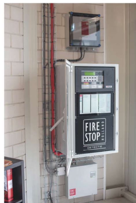
LED paneel in de centrale
