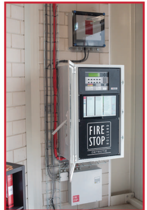
LED paneel in de centrale
